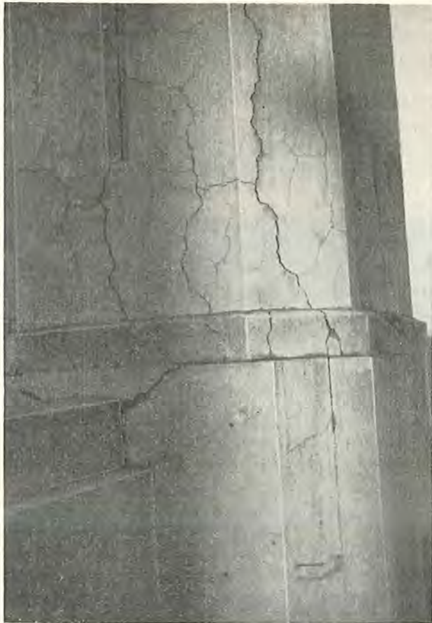
Fig. 2. 18. Revnedannelse i betonpille, Sixth Street Bridge.
